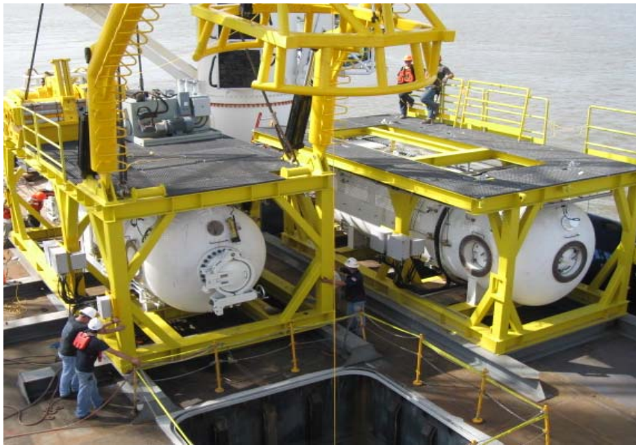
The SAT System is installed on the HARVEY DISCOVERY.
